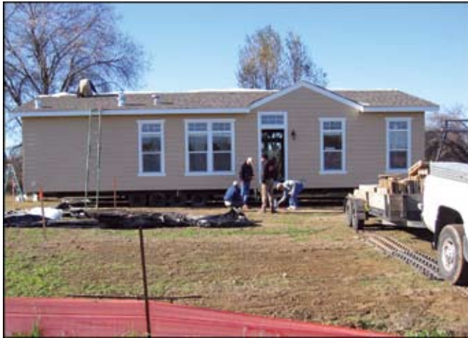
Crews begin setting the HUD home as it arrives from the Fleetwood factory in Woodland, CA.
