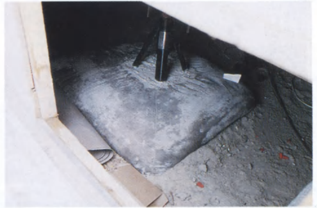
Sure Safe Industries steel/concrete Buttress, 50 of which were placed beneath the Franks' home to stop drywall cracking.
